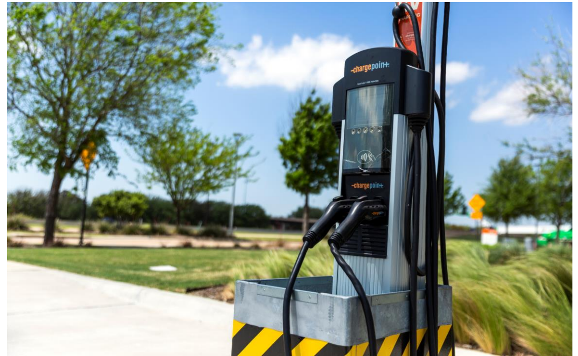
EV Charging Stations
